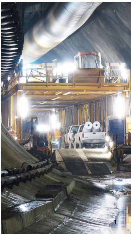
1 Niagara Tunnel Invert carrier / 2 2013 Canadian Project of the Year Award / 3 "Big Becky" cutter head
